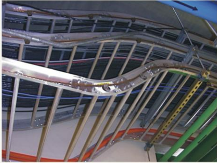
Cable tray and fittings identified for the intended use
